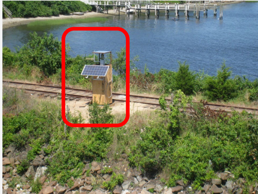
Total station – mounting enclosure with solar engine adjacent to unused railway
